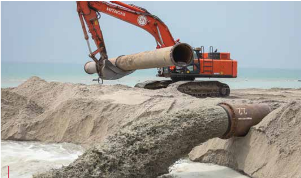
Sand pumped ashore is spread in a controlled way over the area to be reclaimed.
