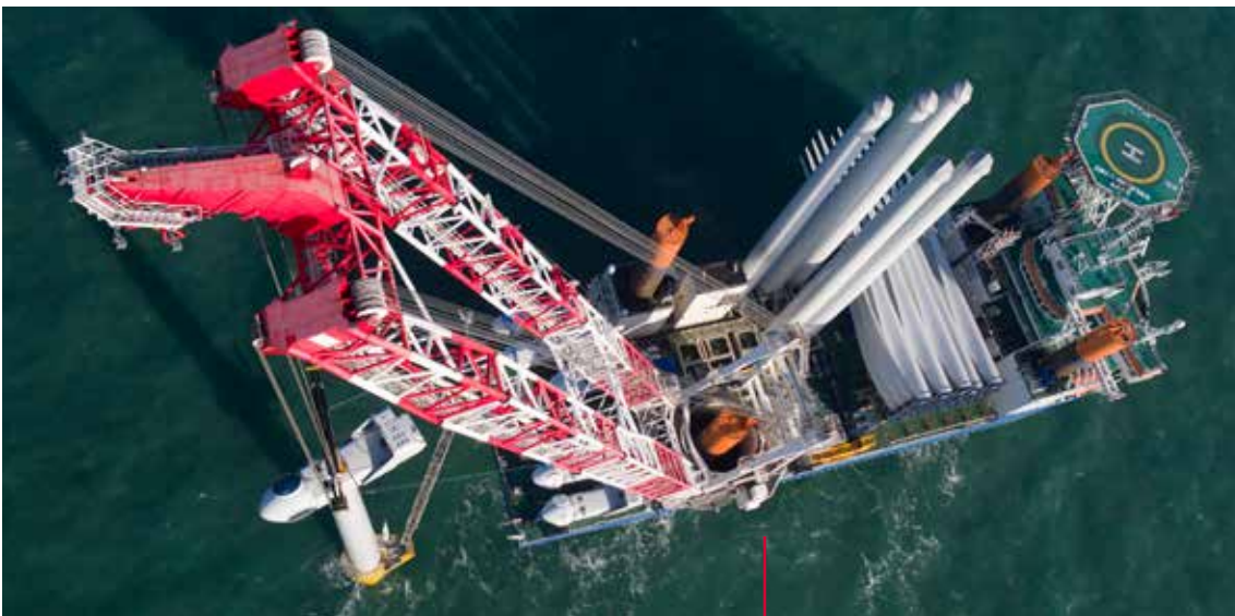
The offshore installation vessel Vole au vent installs wind turbines at sea.
