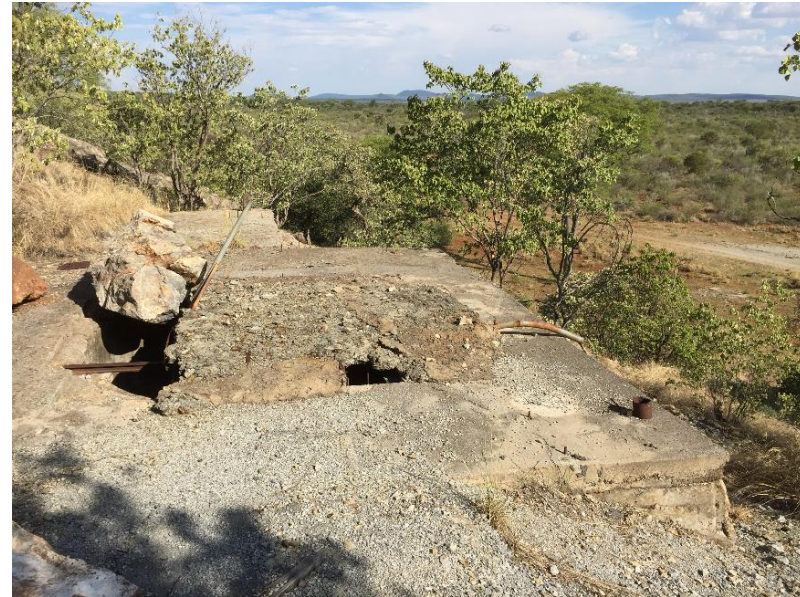
Deblin Mine shaft (approx. 2.5m in diameter and 50m deep) - concrete cover broken and unsafe
