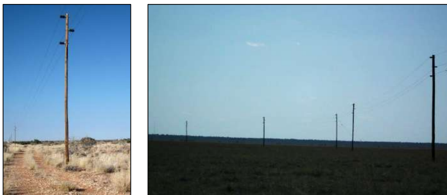
Figure 2. The HPCD (horizontal line post compact delta) structure is used widely for low voltage, private power lines throughout Namibia.
