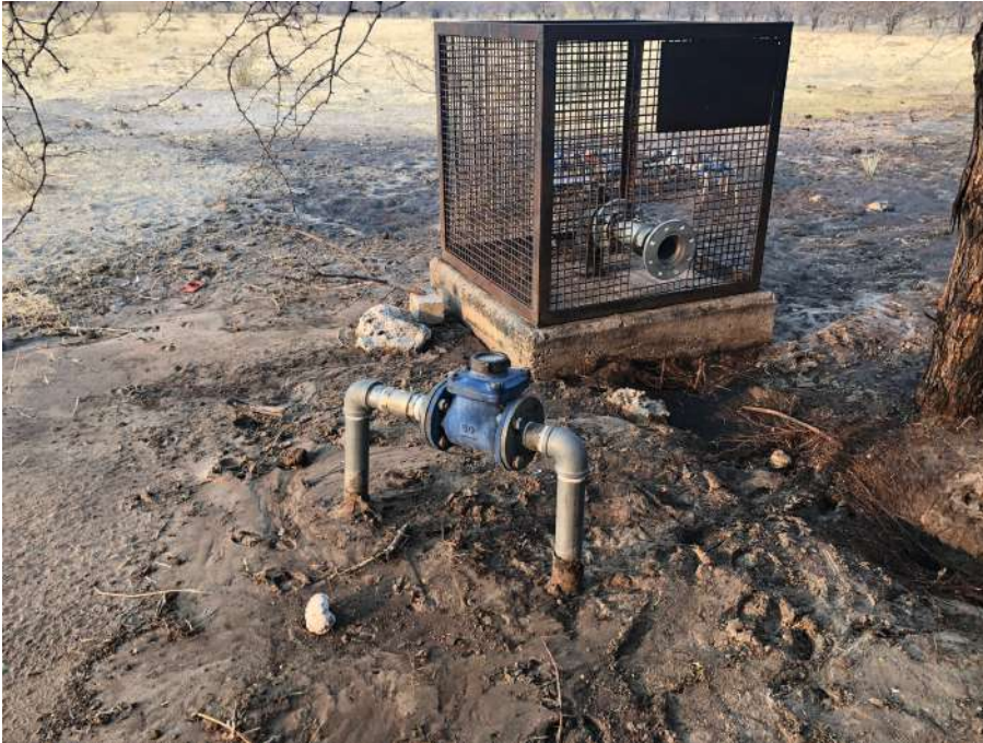
Figure 8: NamWater meter and borehole connection.
