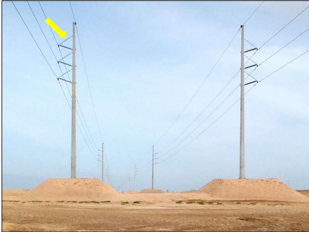
Figure 37. Example of a braced/slanting insulator, where the slope of the insulator may discourage perching by large birds such as vultures, used as a mitigation for electrocutions on the 132 kV steel monopole Kuiseb-Walvis Bay power line.
