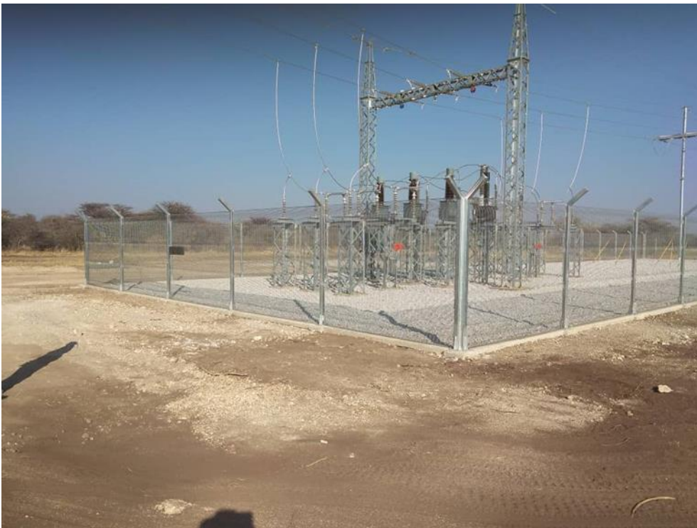
Figure 5 - An example of a metering station
