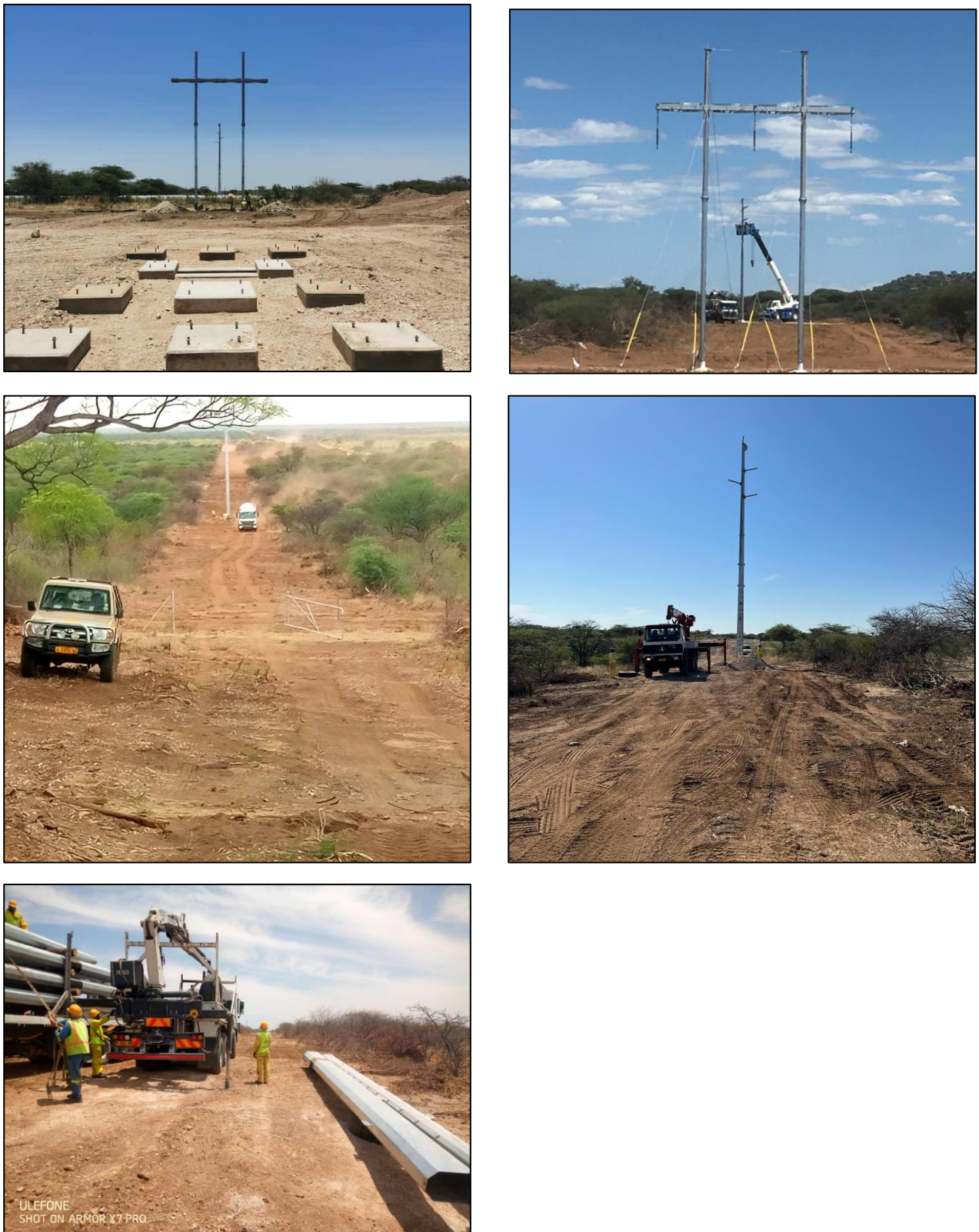
Figure 5. Examples of terminal H-pole structures used at the substation (top left & right); typical construction activities, illustrating the type of disturbance and habitat modification associated with this phase of the project (centre left & right, bottom; photos F de Wet).
