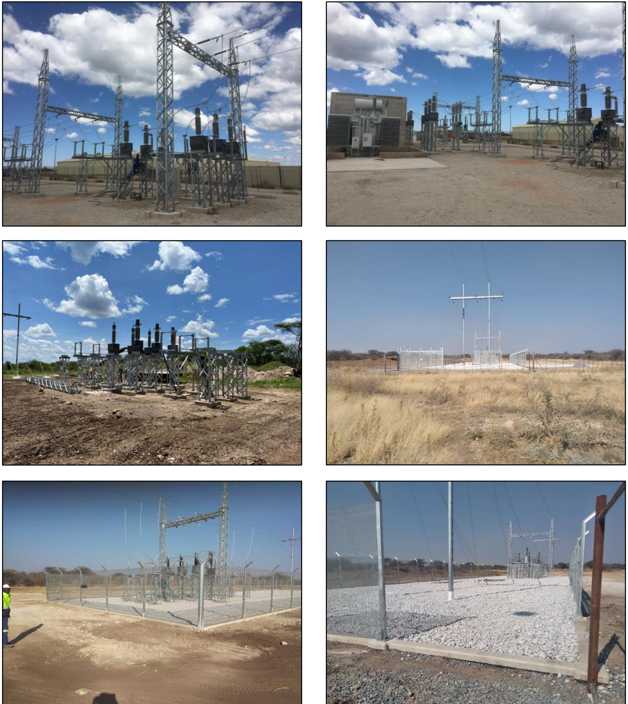
Figure 6. Typical substation and metering structures for the power line (photos F de Wet).
