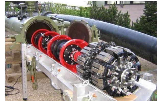
Intermediate Pigging stations are installed at regular intervals
