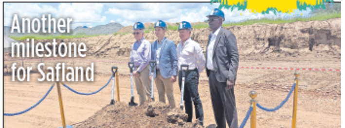
The Safland Property Group recently broke ground for the development of the second-largest distribution centre to be built in Namibia in the last six years.
