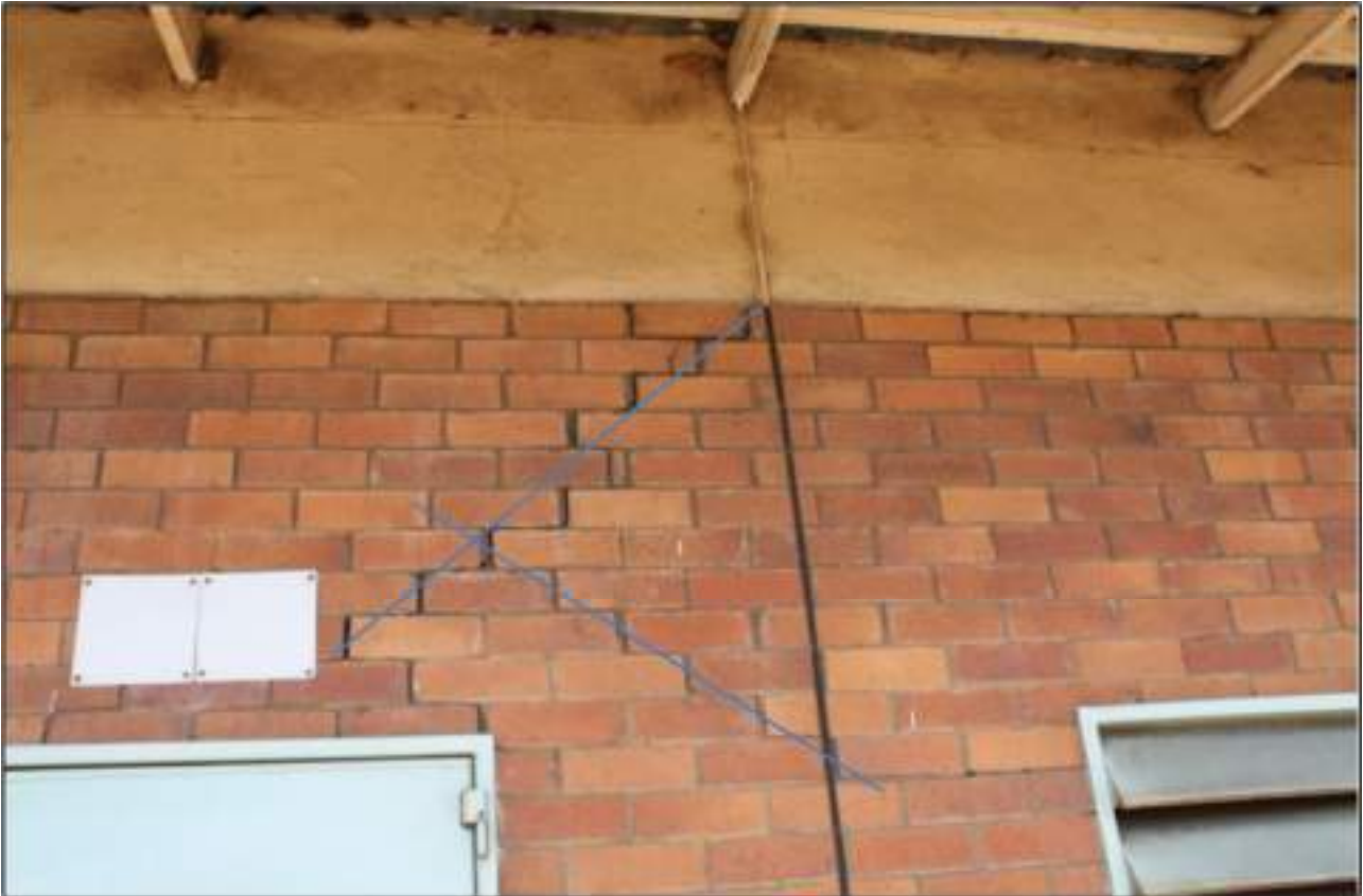
Figure 6: Example of blast induced damage.
