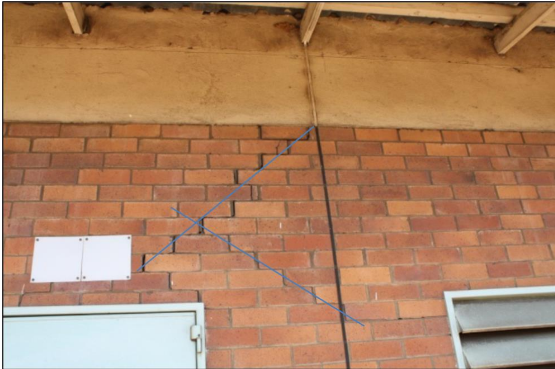
Figure 62 - Example of a typical blast induced damage to a building marked with an X (BMC, 2023).
