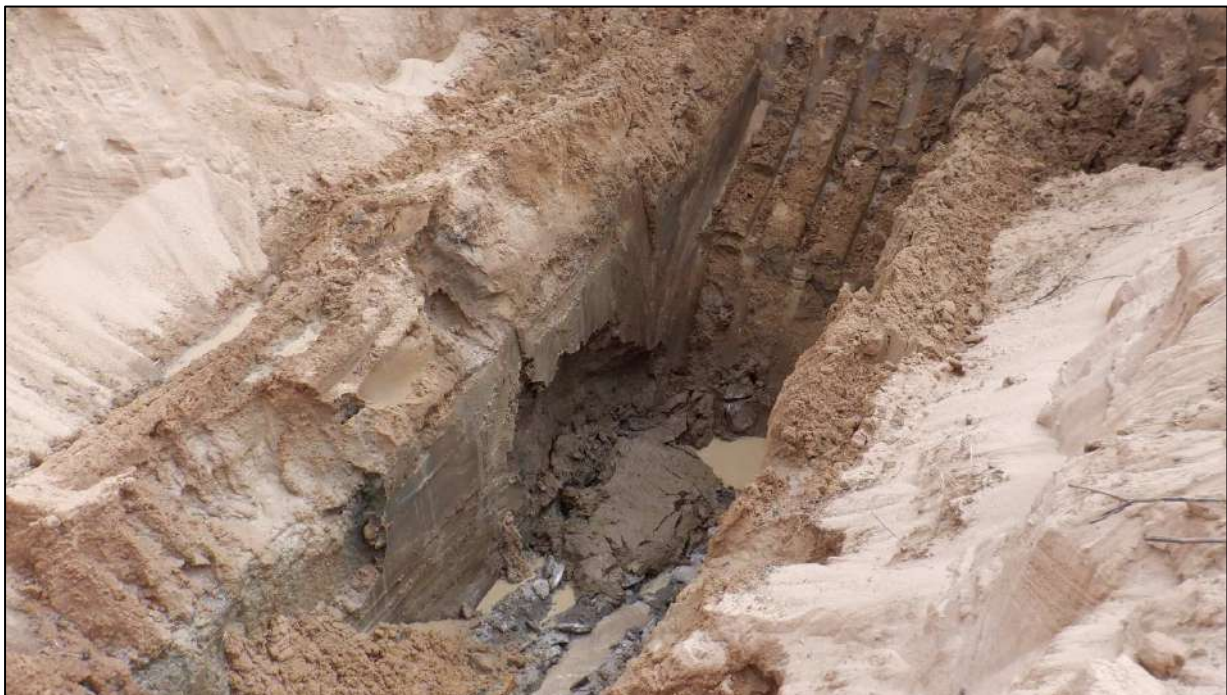
Plate 14: Macro-instability of test pit sidewalls at WRD-TP01.
