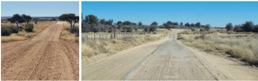
Photos of water course crossing on DR1435 at km 14.5 and concrete drift on DR1535, km 18.9
