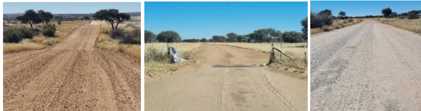
Photos: km 14.5, km 34 and km 34.4 indicating a water course crossing, cattle grid and isolated gravelled sections.
