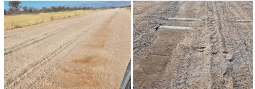
Photos taken on km32 and km40 respectively indicating pavement failure.
