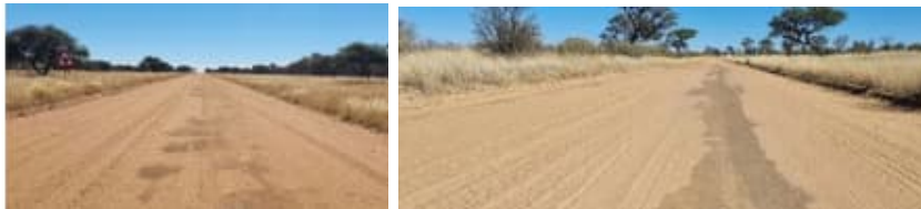
Photos taken on km 21, DR 2166 and km 10.7, MR 53, respectively, indicating the road condition.
