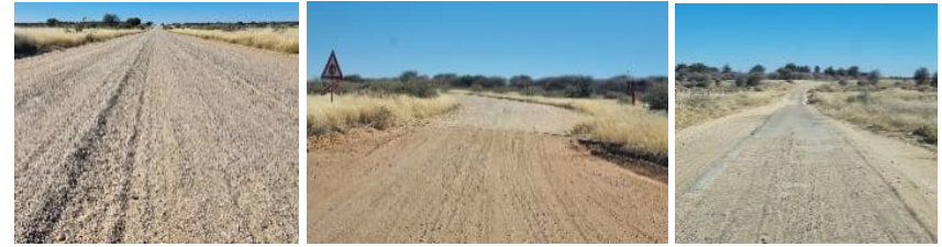
Photos: km 6.8, km 13.8 and km 18.1 indicating minor failures, a rail crossing and a concrete drift.
