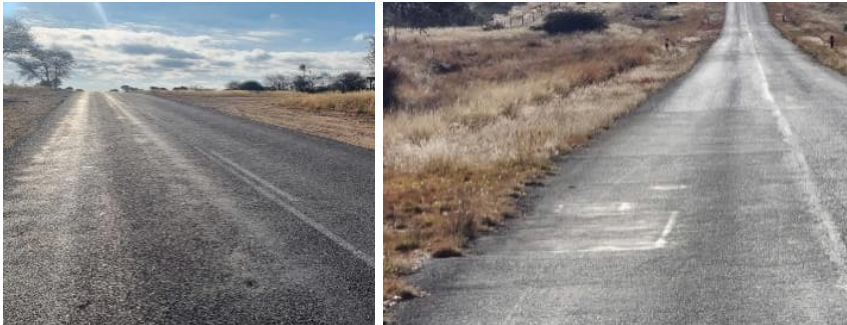
Photos taken at km 1.2 and km 14.7 respectively, indicating the low volume seal pavement and some pothole repairs.
