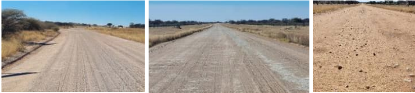
Photos taken on MR59, MR60 and DR2166 respectively, indicating material on sections of these roads.
