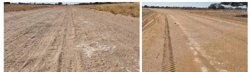
Photos taken on MR60 at km 17.5 and km 43 respectively indicating the road condition.
