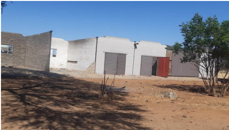
Figure 5. Top Photograph: Weather station and weather instruments within ML197. Bottom photograph Uninhabited burnt Farmstead ruins within the same precinct.
