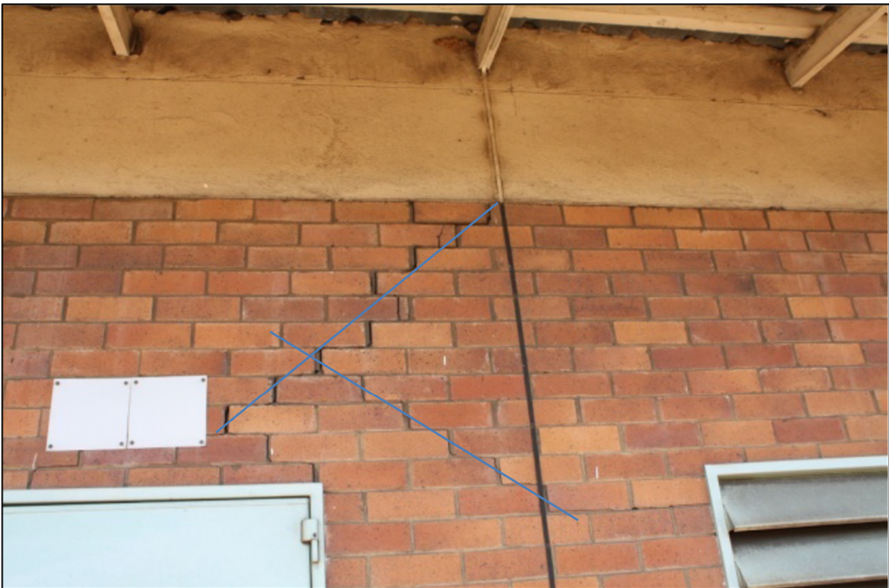
Figure 7: Example of blast induced damage.
