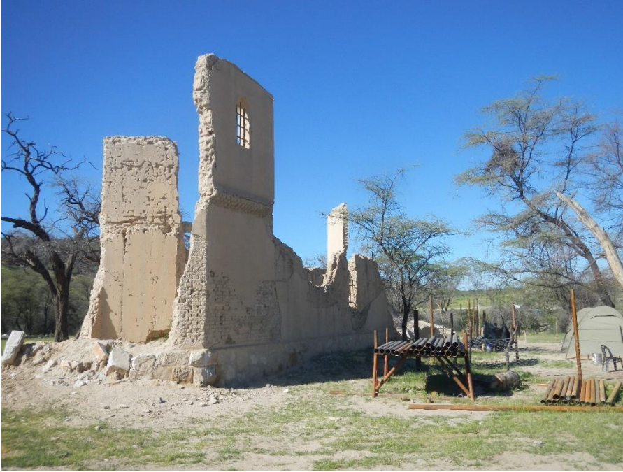
Figure 8: Okawayo 480, encroachment of driller's camp on heritage building.
