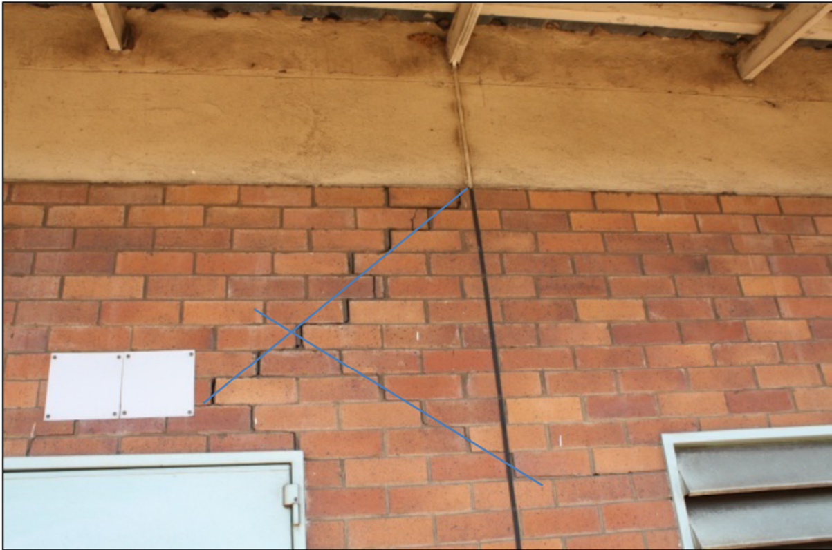
Figure 8: Example of blast induced damage.
