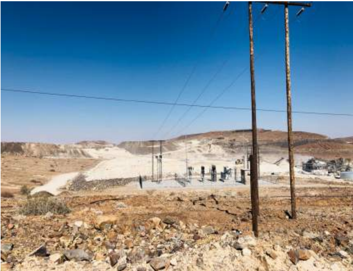
Figure 9 - Main power supply off take (Source: ECC, 2021)
