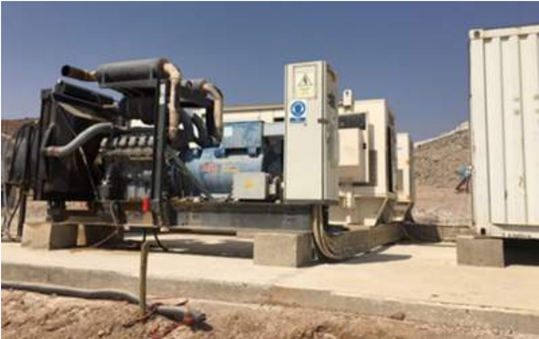
Figure 10 - Genset stand-by power source (Source: Minxcon, 2021)
