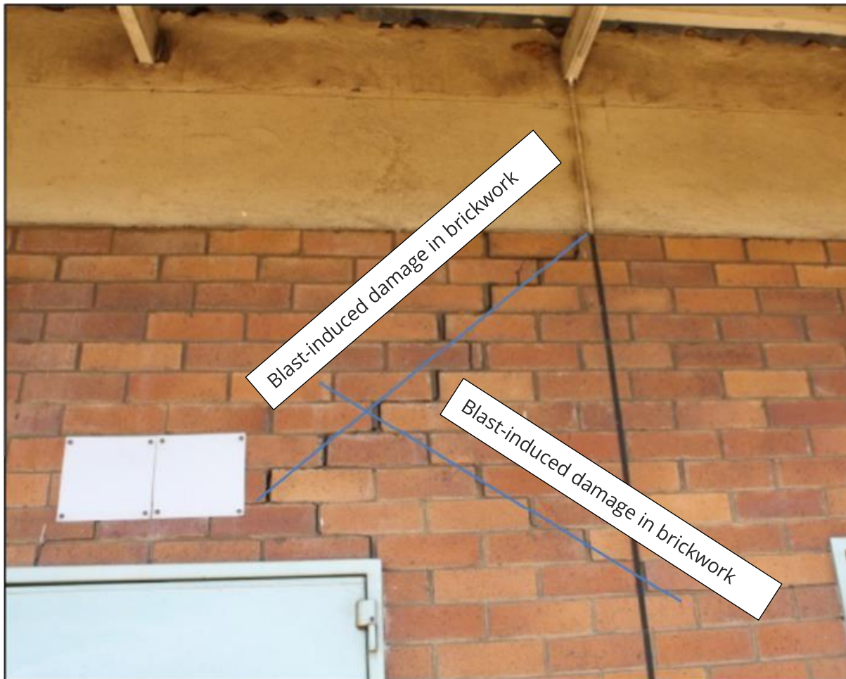
Figure 15 – Example of blast-induced damage
