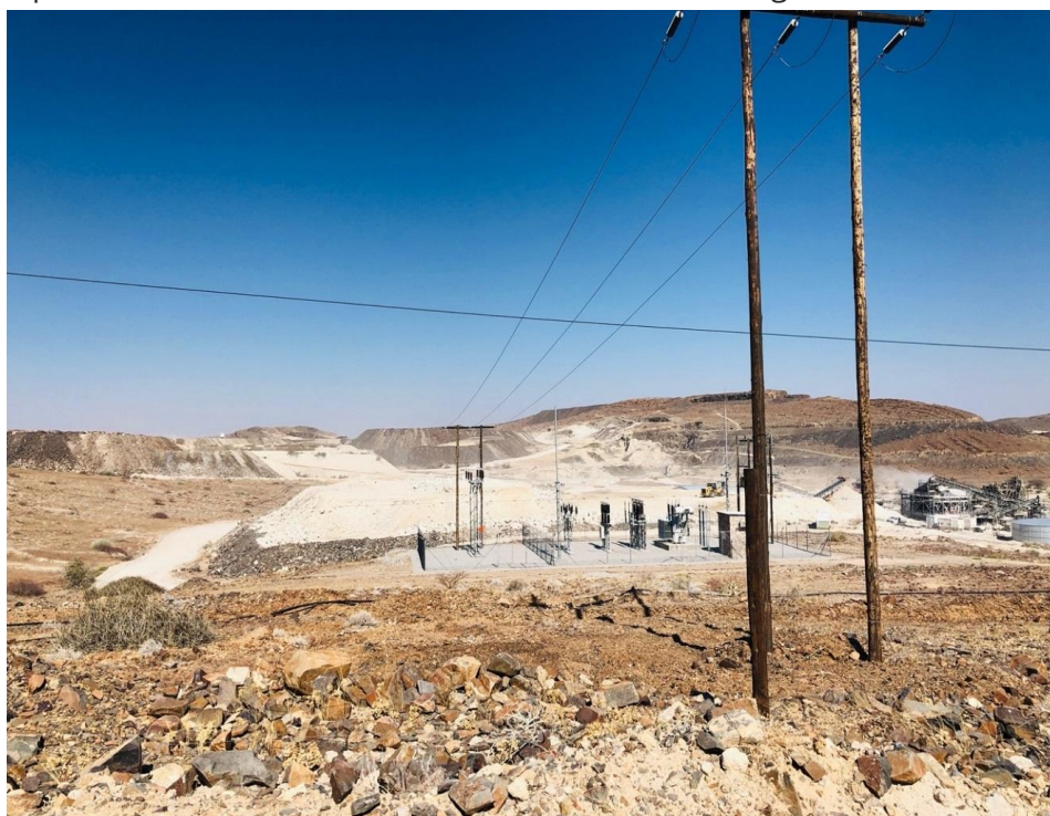
Figure 21 - Main power supply off-take (Source: ECC, 2021)
