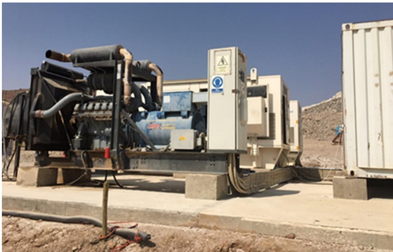
Figure 22 - Genset stand-by power source (Source: Minxcon, 2021)
