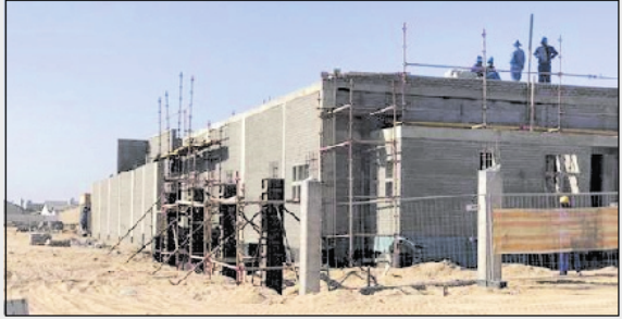
The Paratus landing station will host the Equiano undersea cable system transmission equipment. PHOTO: K. J. J. J.
