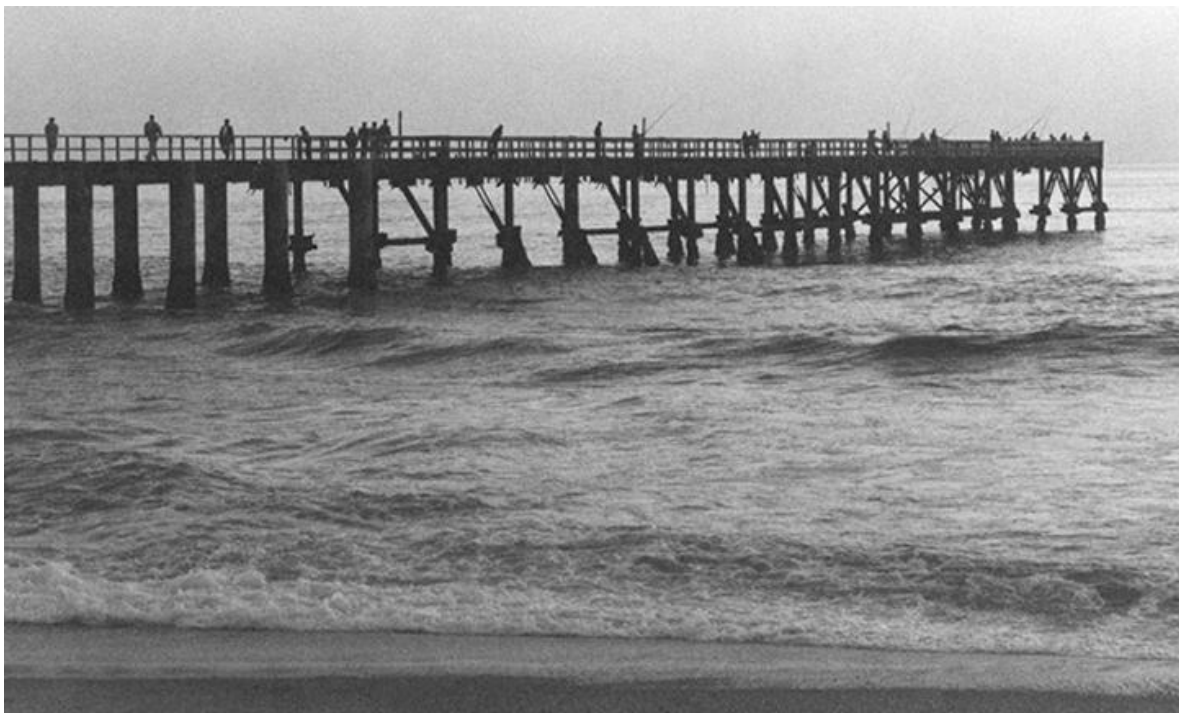
The rusted steel jetty (app. 1960), used by fishermen and people who took a walk there.
