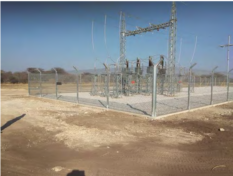
Figure 5 - An example of a metering station
