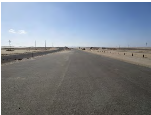
Figure 35 - Photo taken on a section of the D1984 road (Source: Zutari, 2024)
