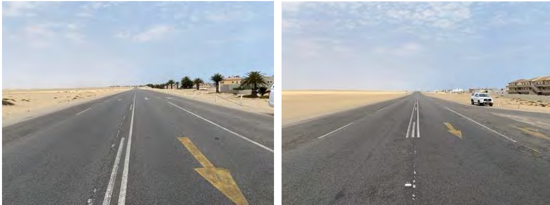
Figure 34 - Photos taken on a section of the B2 road (cracks and potholes) (Source: Zutari, 2024)
