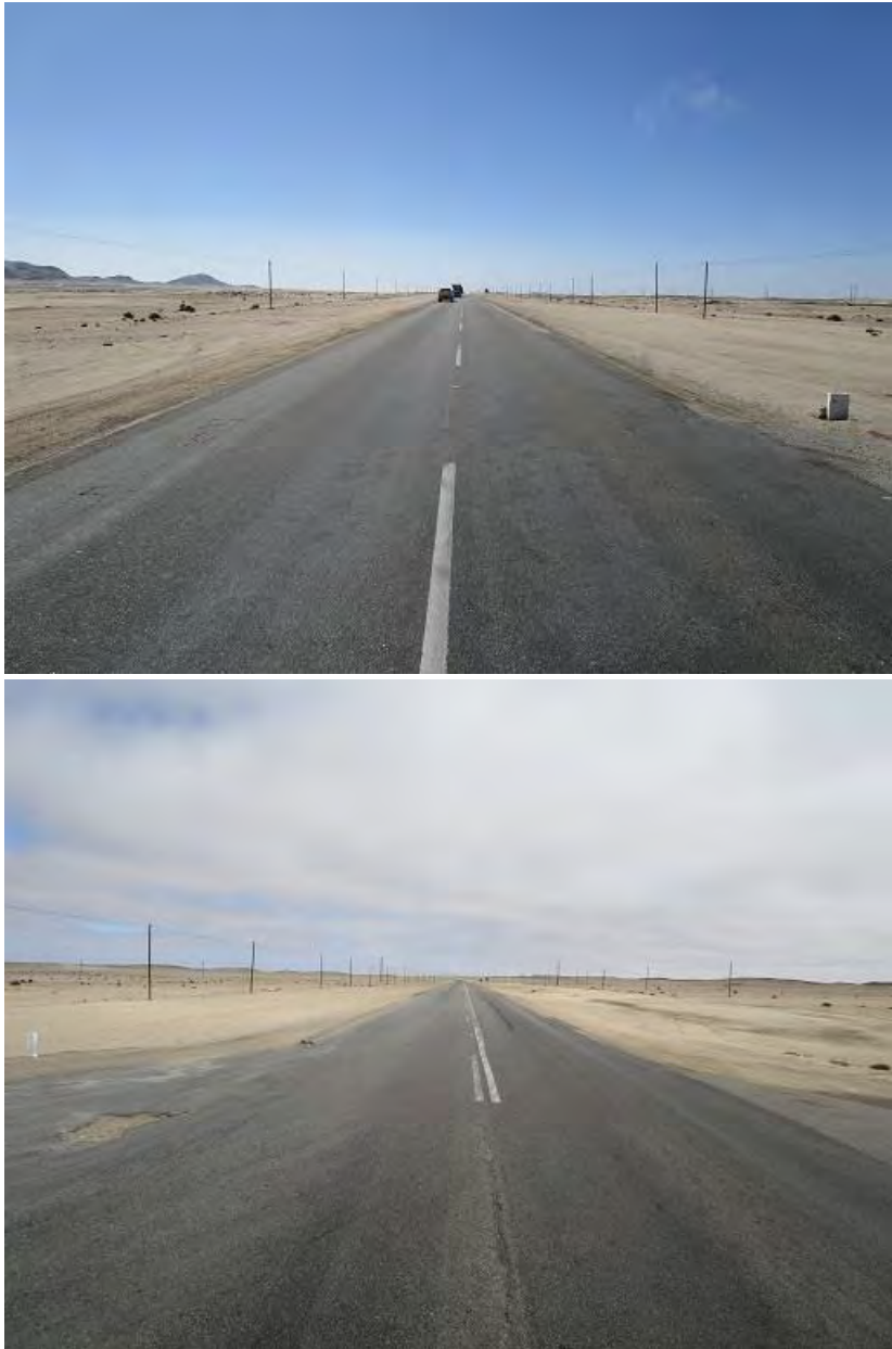
Figure 23 - Photos taken on section of the B12 Road (cracks and potholes) (Source: Zutari, 2024)
