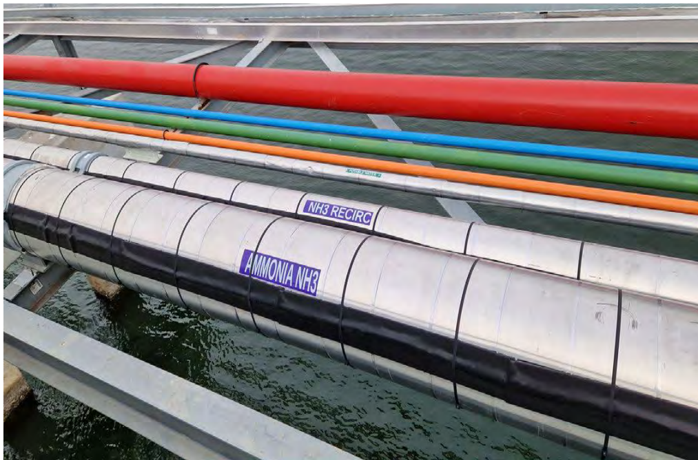
Figure 4: A typical example of the ammonia pipeline above the ground. Image credit: (ECC, 2024).
