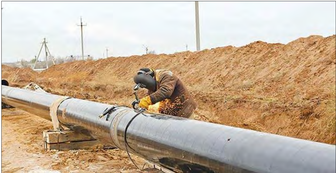
Figure 5: A typical example of the ammonia pipeline above the ground envisioned for the 80km route between Walvis Bay and Arandis. Image credit: (ECC, 2024).
