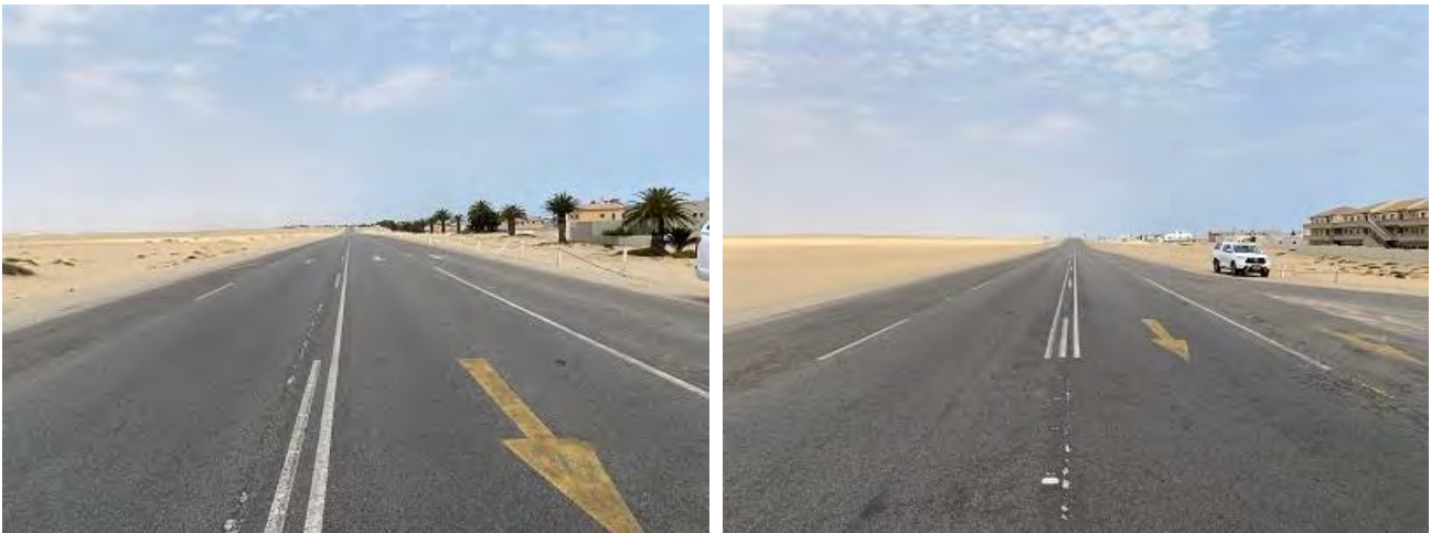
Figure 8 – Photos taken on section of the B2 Road (Cracks and Potholes)
