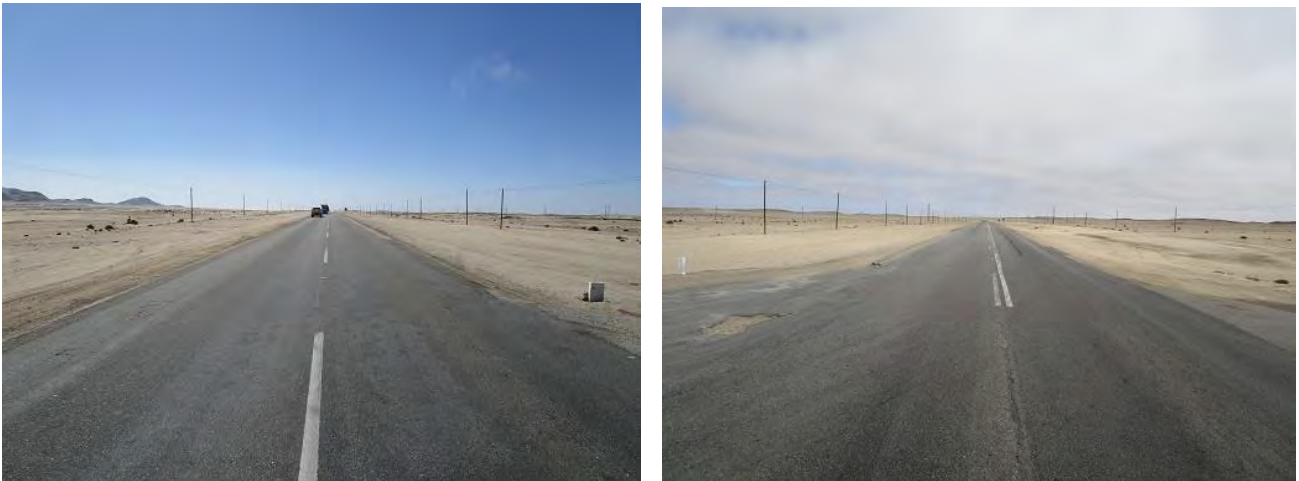
Figure 9 – Photos taken on section of the B2 Road (Cracks and Potholes)
