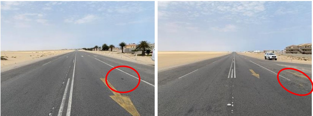
Figure 9 – Photos of minor defects taken on a section of the B2 Road
