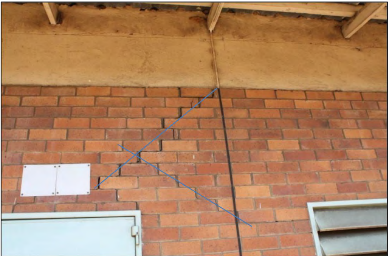
Figure 7: Example of blast induced damage.
