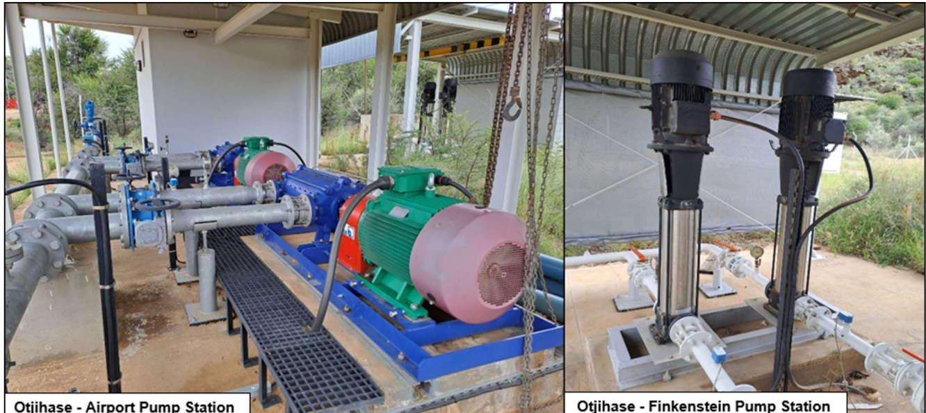
Figure 11: Otjihase - Airport and Finkenstein pumps.
