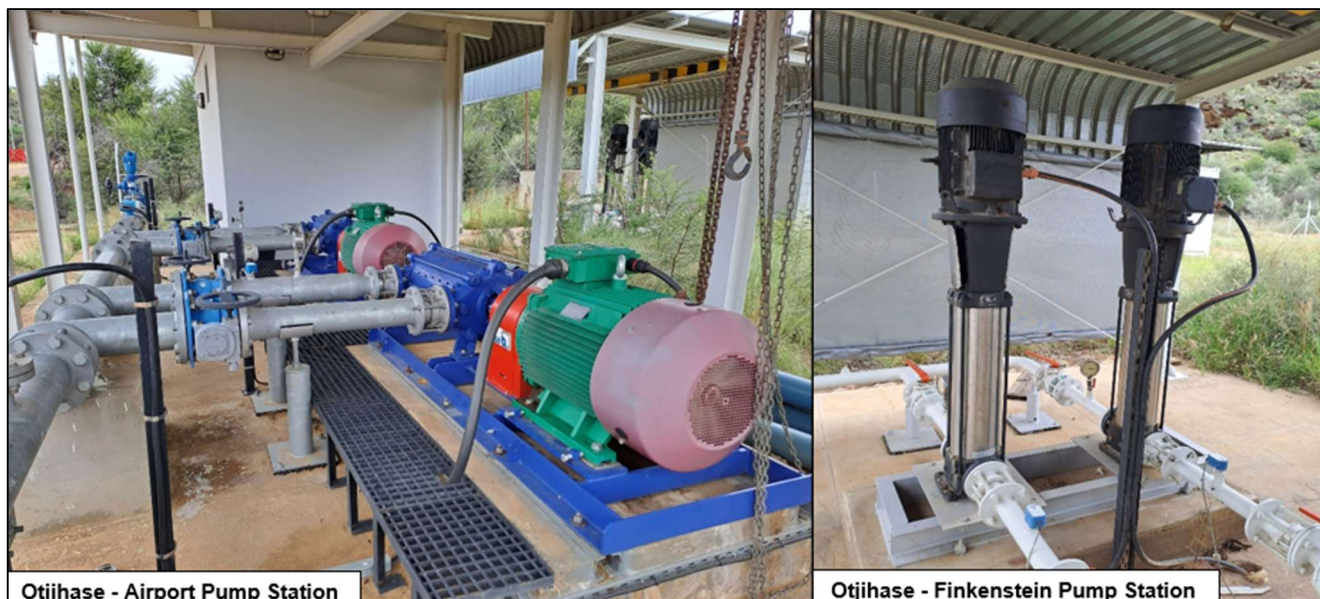
Figure 11: Otjihase - Airport and Finkenstein pumps.
