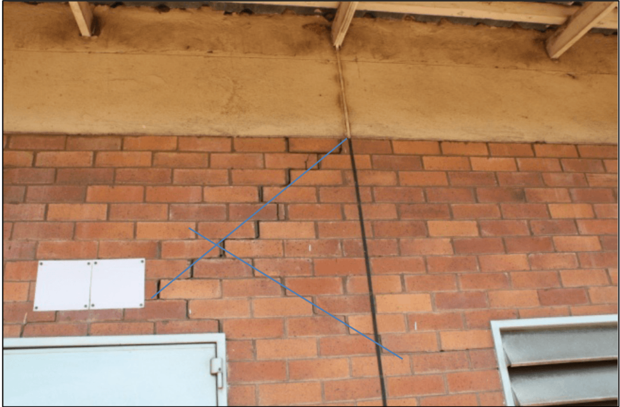
Figure 52 - Example of a typical blast induced damage to a building marked with an X (Source: BMC, 2023).
