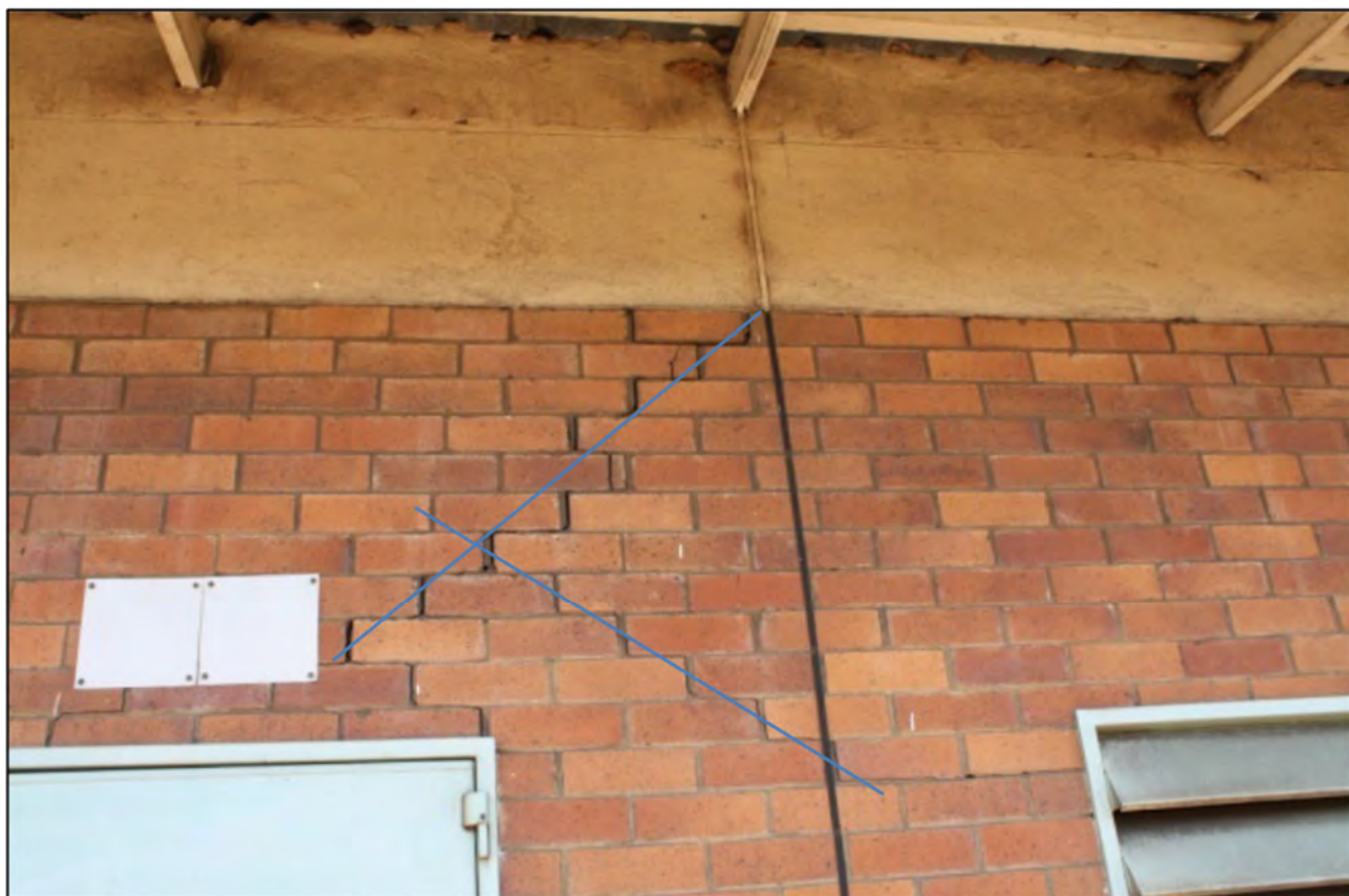
Figure 7: Example of blast induced damage.
